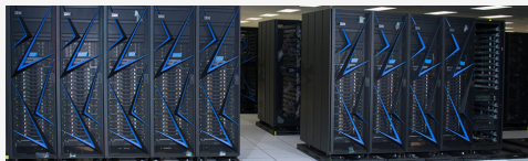
Figure: Sierra supercomputer in Livermore California.
